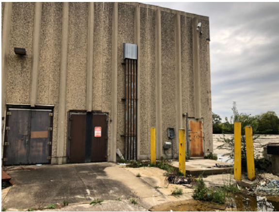
11 ELECTRICAL PIPING - NORTH
